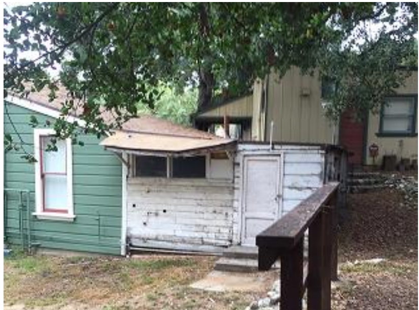
Shed at the back of Richardson House, showing deterioration. Lizzie's Trail Inn to right. (photo by Maggie Ellis)
